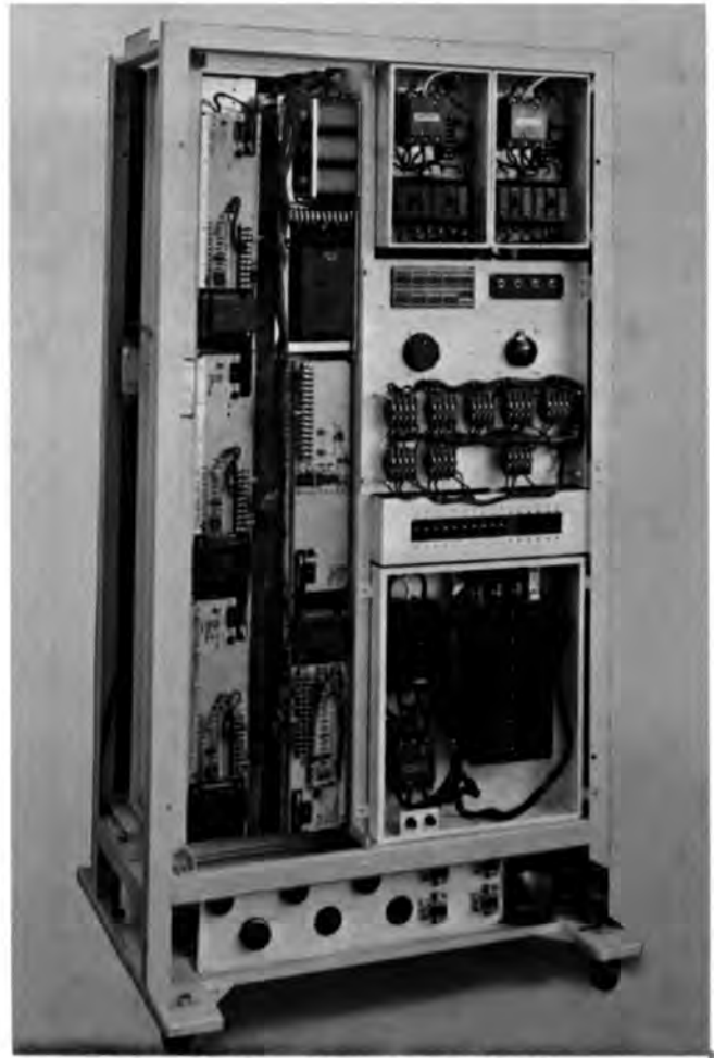
Figure 17. Universal Frame, Power Supply Mounting (Front View)
